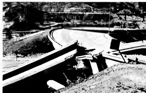
Photo 12. Damaged overcrossing at the Golden State Freeway and Foothill Freeway interchange [4].
